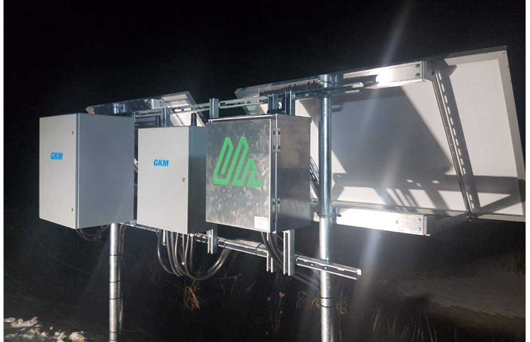
Fully commissioned datalogger
